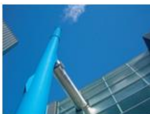
Flue gas treatment
